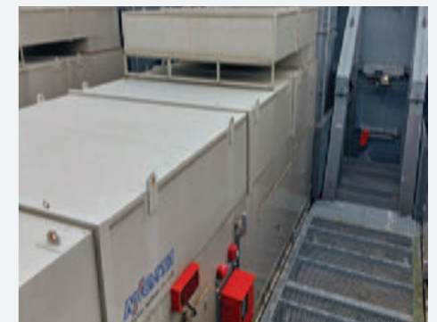
Gas Turbine Generator
