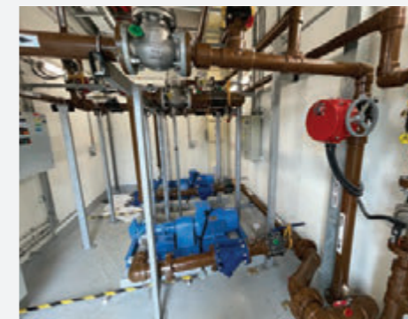
Fuel Transfer System
