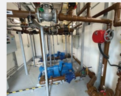
Fuel Transfer System
