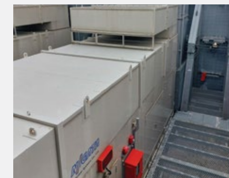
Gas Turbine Generator
